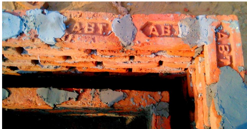
Fig 10: Gap between inner and outer wall
