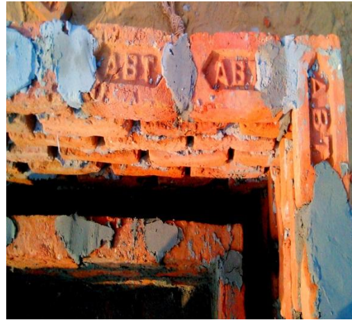
Fig 5: Gap between outer wall and inner wall
