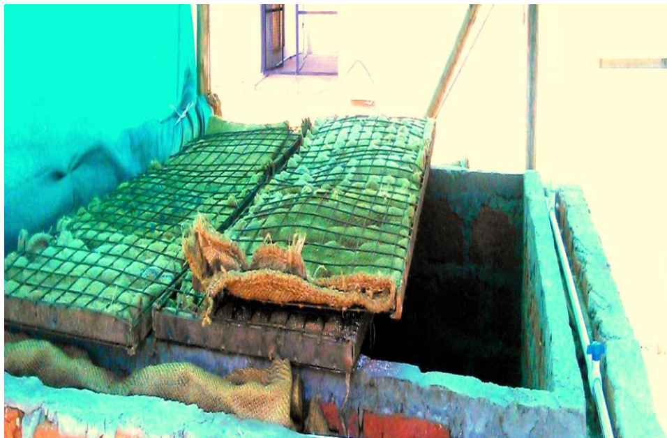
Fig 6: Gates are placed on cooling chamber
