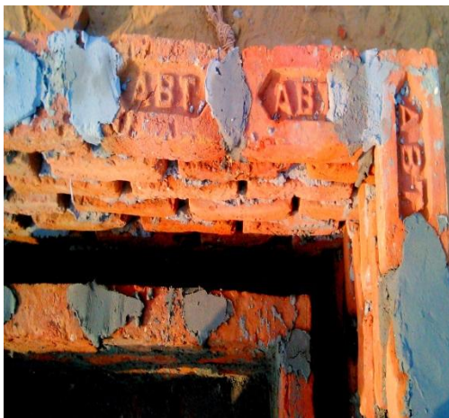
Fig 5: Gap between outer wall and inner wall
