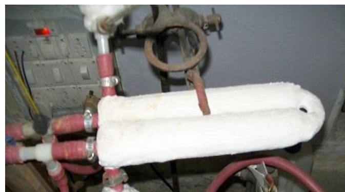
Fig 2: Installed double tube Hair-pin heat exchanger in laboratory.
